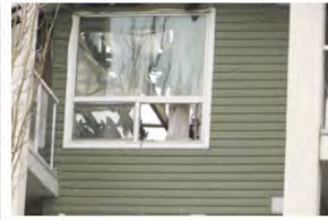
ANNA BOROWIECKI/CAPTION Torned rafters and a tattered curtain blow across a broken window after the morning after a massive fire destroyed Citadel Mews West.
